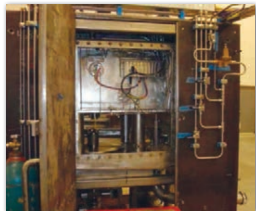
AVANTech Fabricated Shielded ASX Transfer Station
