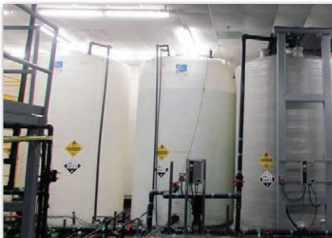
Tank Waste Simulant Storage Tanks
