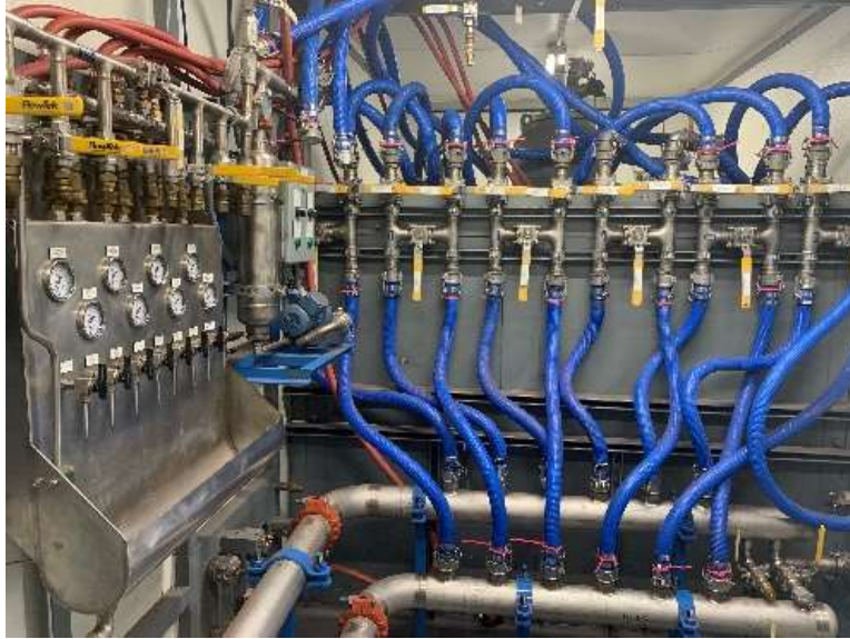
Fig. 4. WPS System Manifold System
