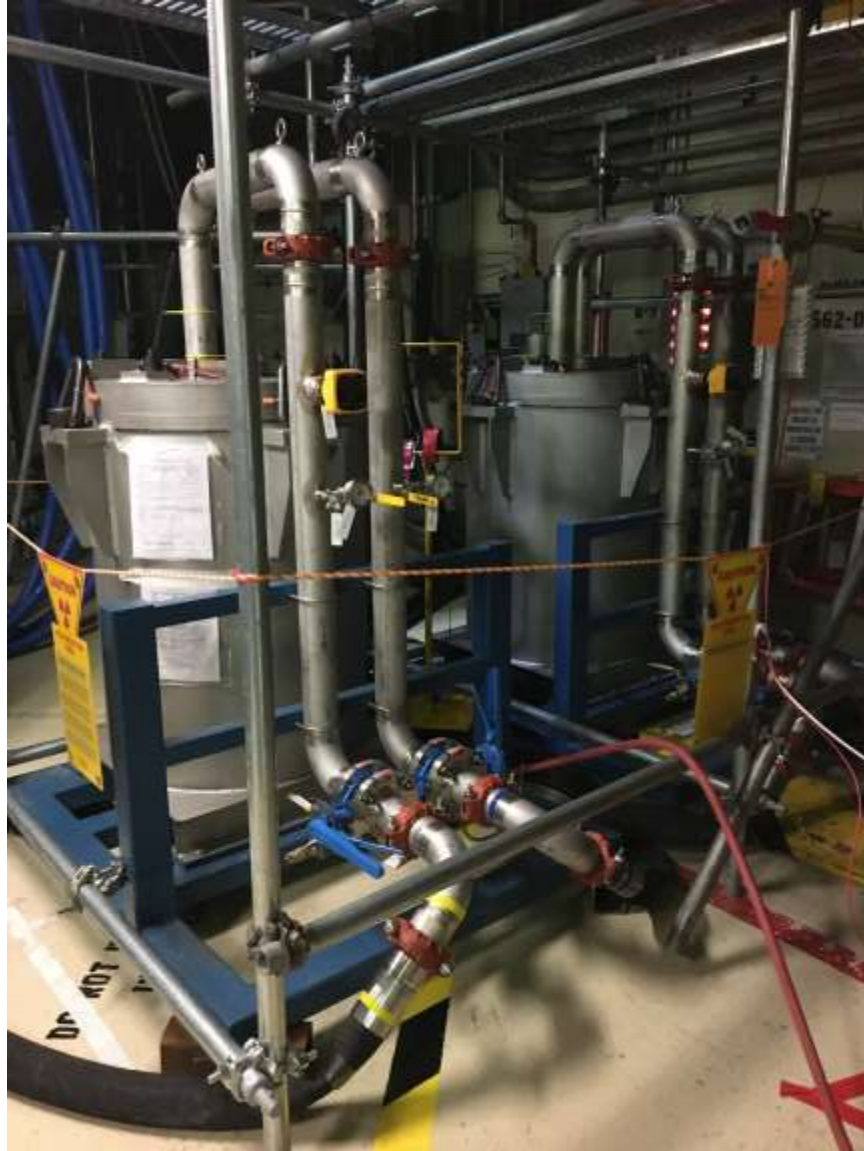
Fig. 1. Reactor Building, SW Basement, Torus Filtration Setup
