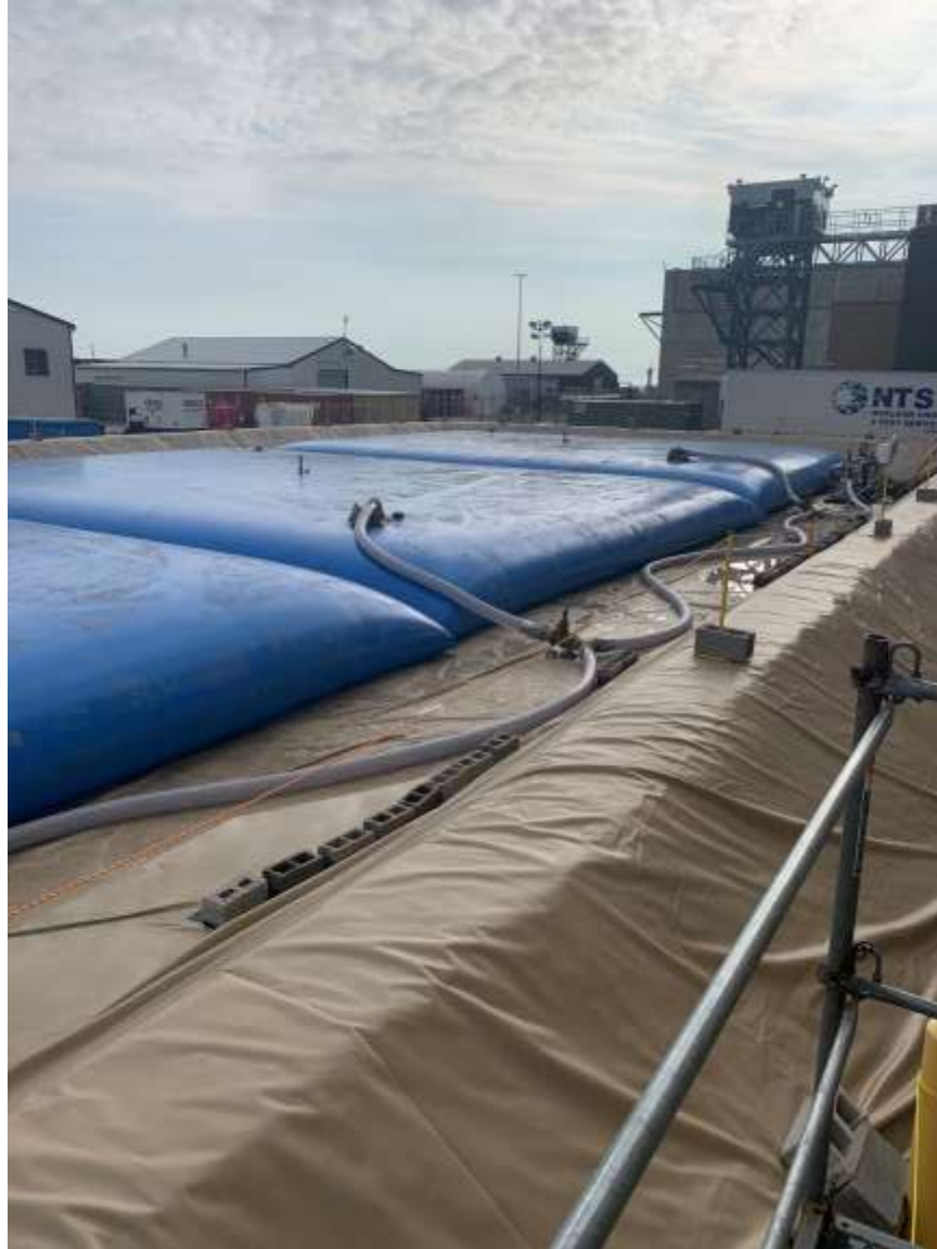
Fig. 3. Torus Water Storage Post-Filtration
