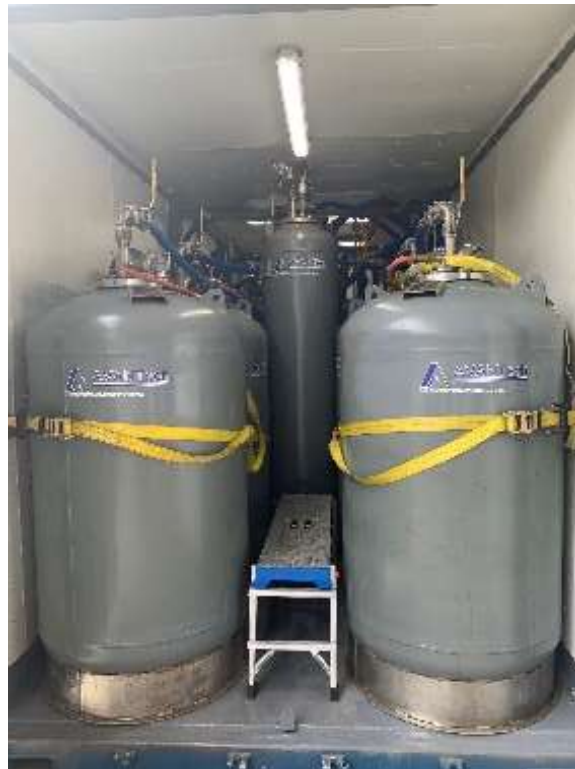
Fig. 5. WPS Ion Exchange Vessels
