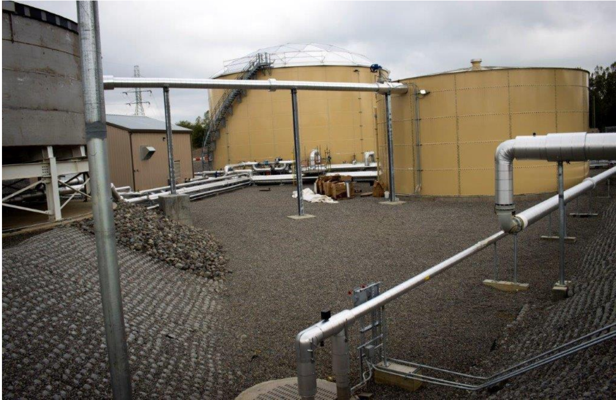
Figure 4. ILTS Pretreatment Equipment
